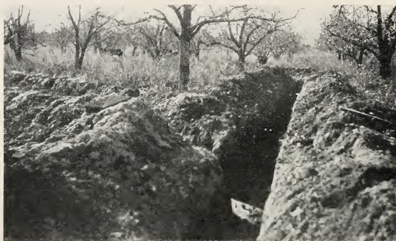
Fig. 14.—Box drains in place and ready for backfilling in a Placer County pear orchard.
